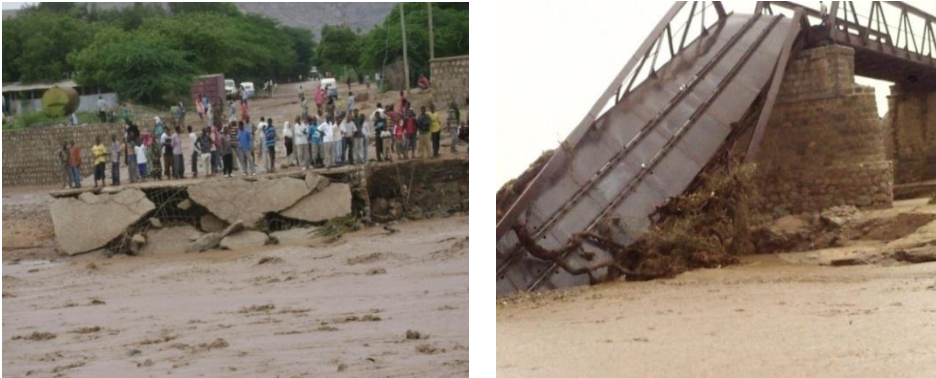
Figure 3.13: Flood Damage on Hafkat ford and Damage on Railway Bridge
