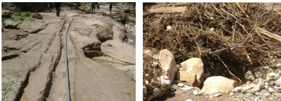
Figure 3.10: Flood damage on potable water pipe lines
