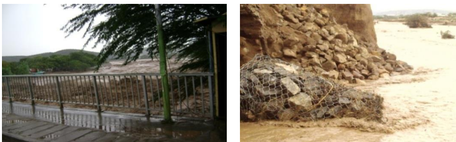
Figure 3.11: Water level around Kezira main Bridge & Damages on gabion
