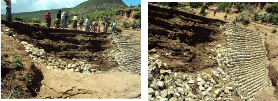
Figure 3.12: Damage on Sediment Storage Dams(SSDs) or damage on infrastructure
