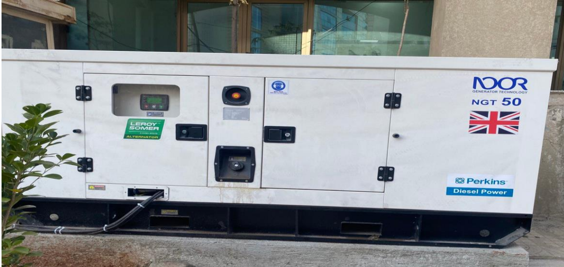
Picture 4: New Generator purchased
